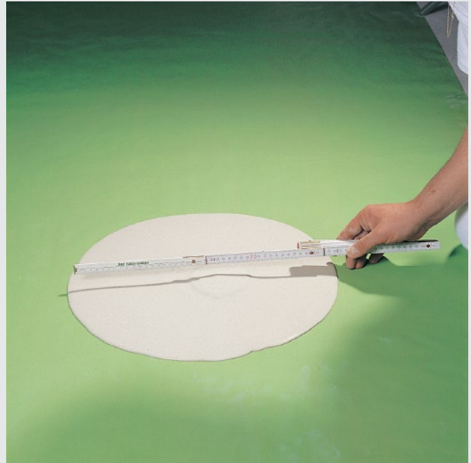
Stay within the defined flow-slump value. The screed may not lose water during application.
