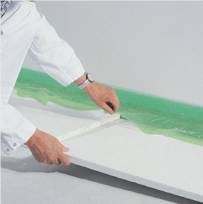
Slide EPS insulation underneath the foil of the edge insulation strip and apply row by row
